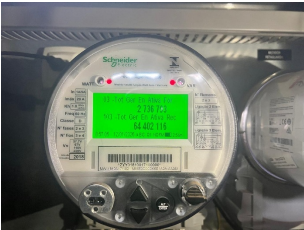
Meter 3 (UTE 2 – Central Energética Tupaciguara - Main)
