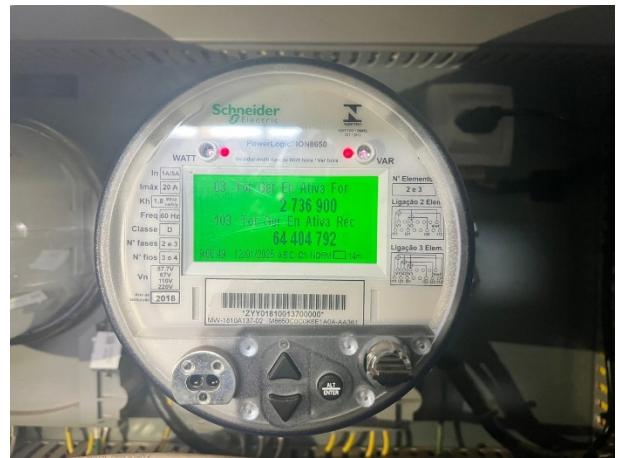
Meter 4 (UTE 2 – Central Energética Tupaciguara - Check)
